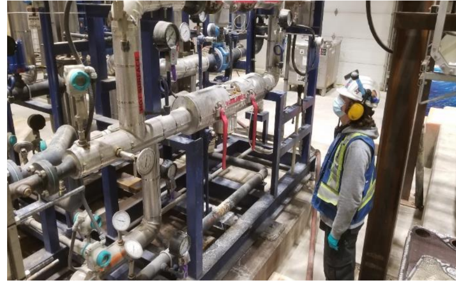
Stripping Circuit Heat Exchanger
