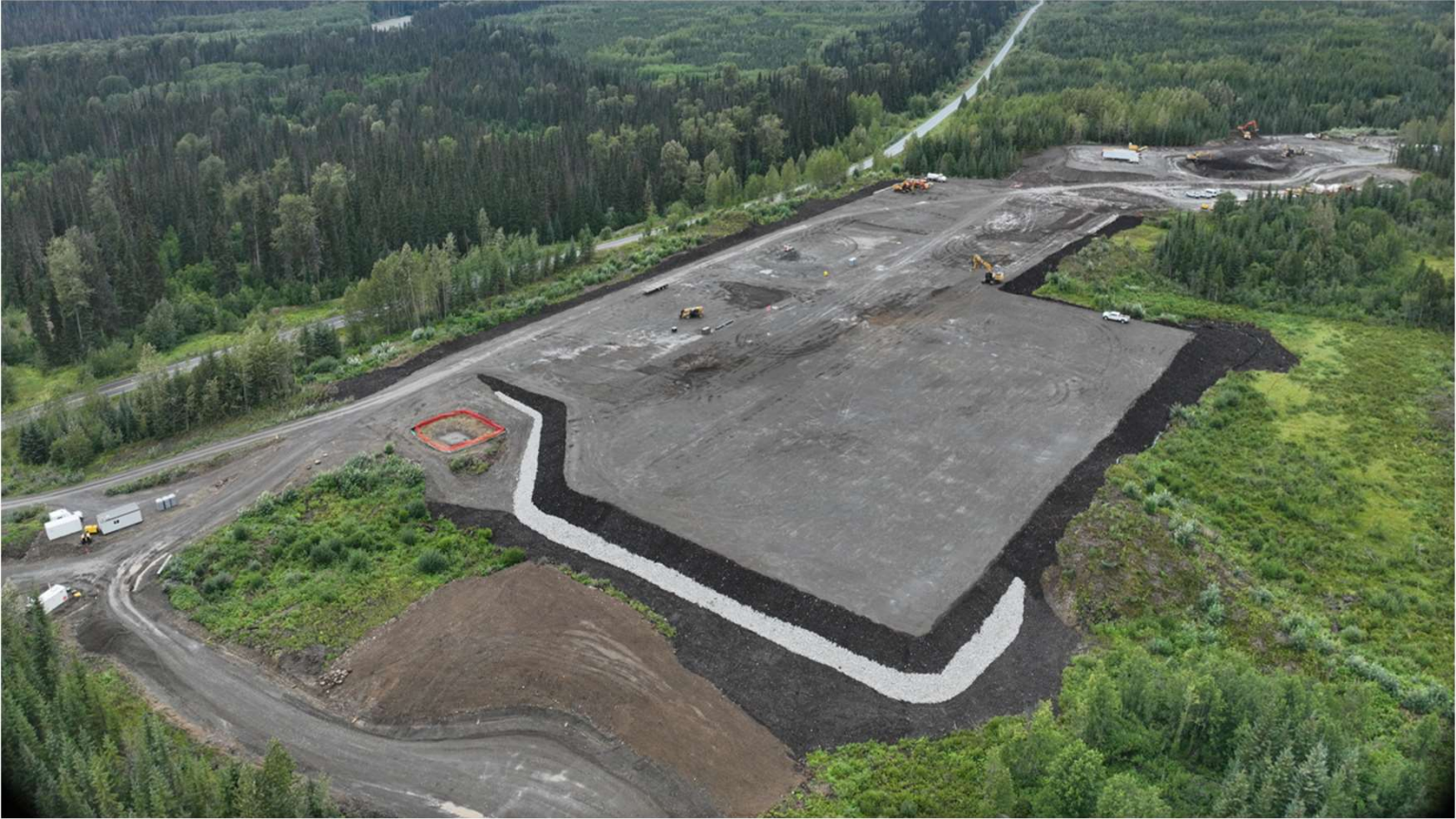
BC Hydro's Treaty Creek Terminal
